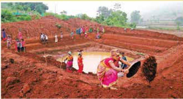
The inhabitants of Uppergodi village are engaged in construction work of Farm Pond
